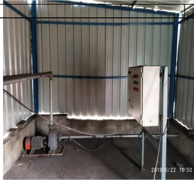
Control panel and Pump
