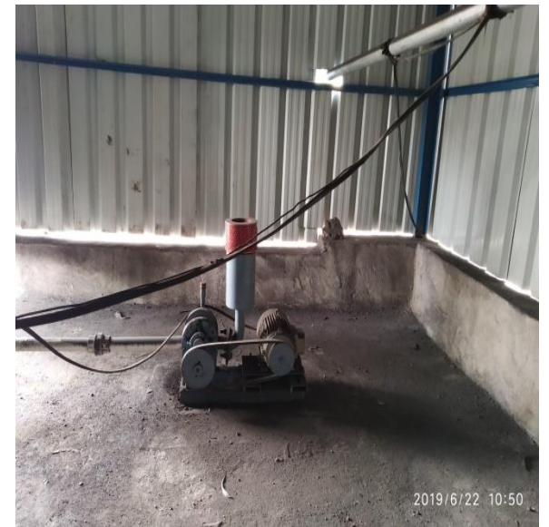
Compressor for Aeration
